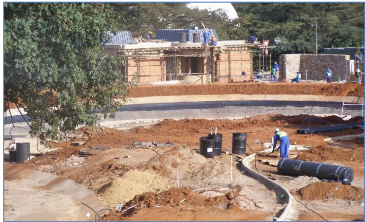
Excavation & construction of the area to be lined with the Sealmac® Dam Lining System
